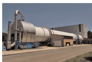
Installation de compostage
